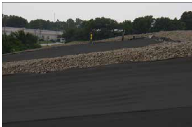
Landfill Odor Control Barrier
