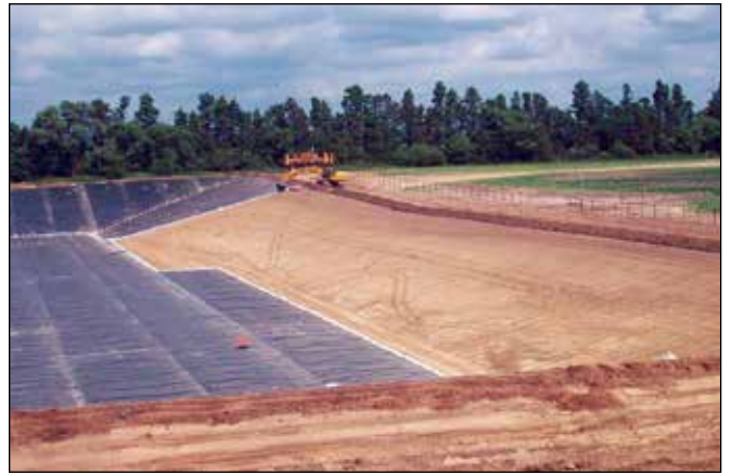
Reservoir Containment Liner
