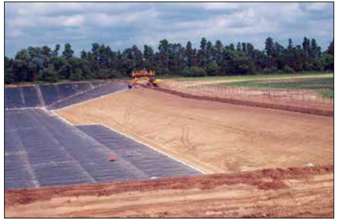
Reservoir Containment Liner
