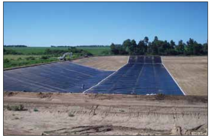
Waste Lagoon Liner
