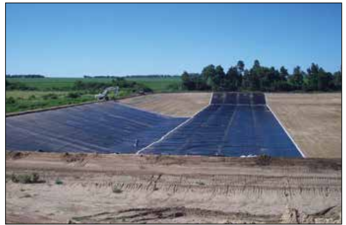
Waste Lagoon Liner
