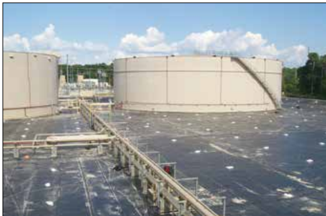
Tank Farm Secondary Containment
