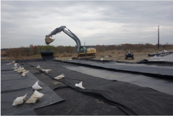
Placement of factory assembled DuraSkrim® K45BT2 panels on top of prepared platform.
