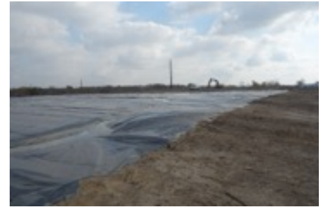
Solutia Landfill: Installation of factory assembled DuraSkrim® R20BV panels over exposed sludge.
