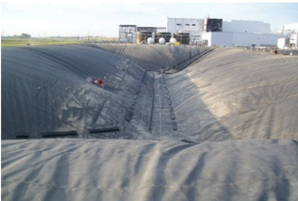
Cover testing with inflation to check for any damage prior to filling
