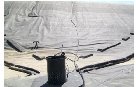
T vent and pump housing
