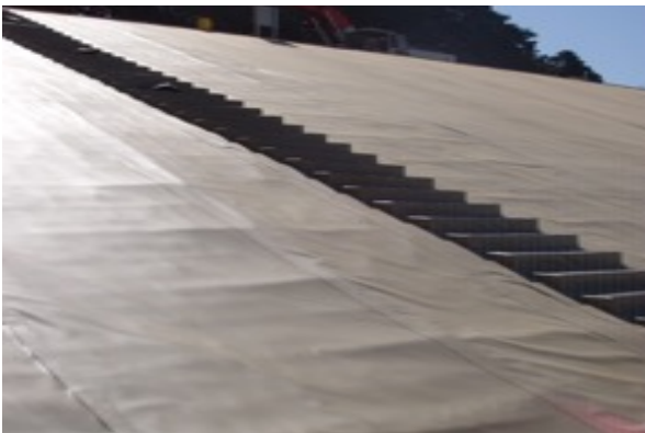
Access stairs on cover – built from foam and wrapped in RPP cover material
